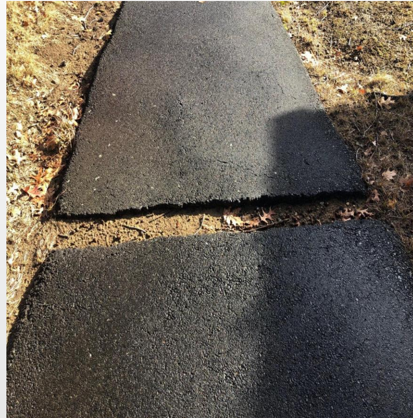
Tripping Hazards in Sidewalks
