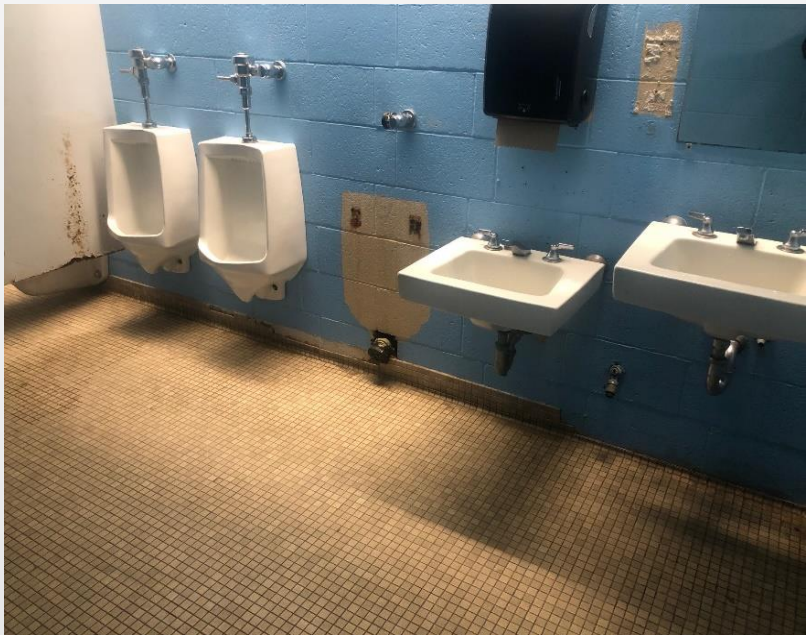
Missing Plumbing Fixtures
