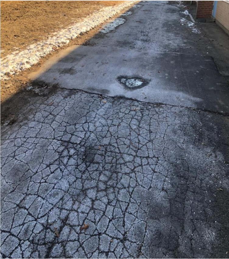
Deteriorating Paving at Play Areas
