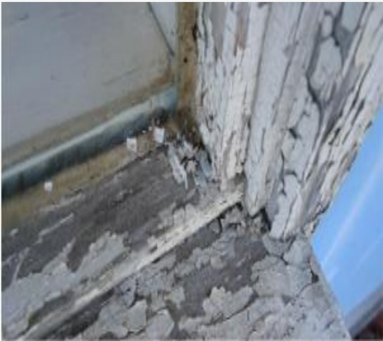
Deteriorating Window Framing
