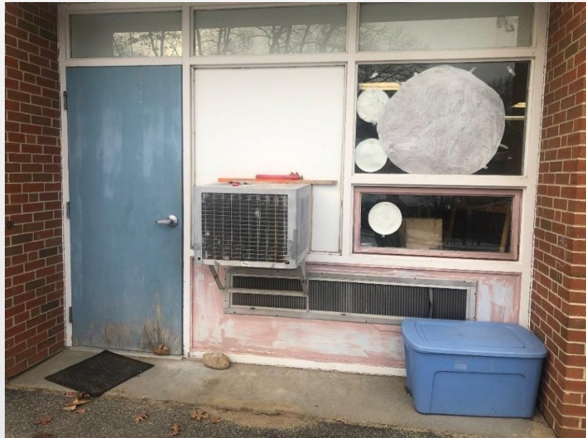
Lack of Natural Light/Ventilation
