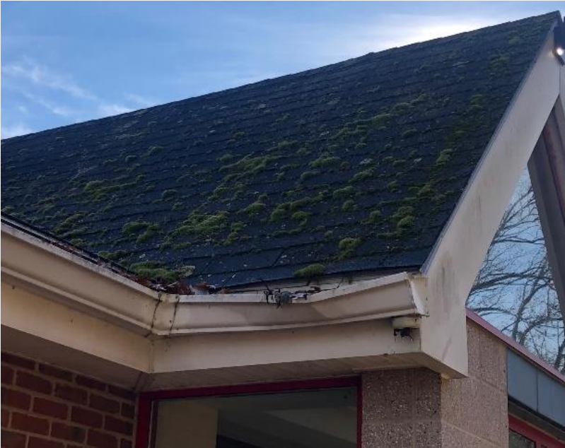
Deteriorating Roof/Damaged Gutters
