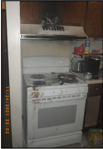
Damage at property where Fire Stop product activated
