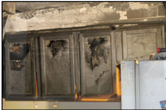
Damage from cooking fire without Fire Stop activation. Fire was able to spread freely prior to WAFD arrival
