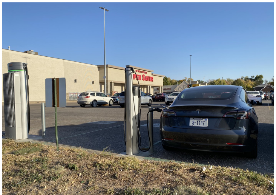
EV Charging Station, Grand Island Source: Marvin Planning Consultants
