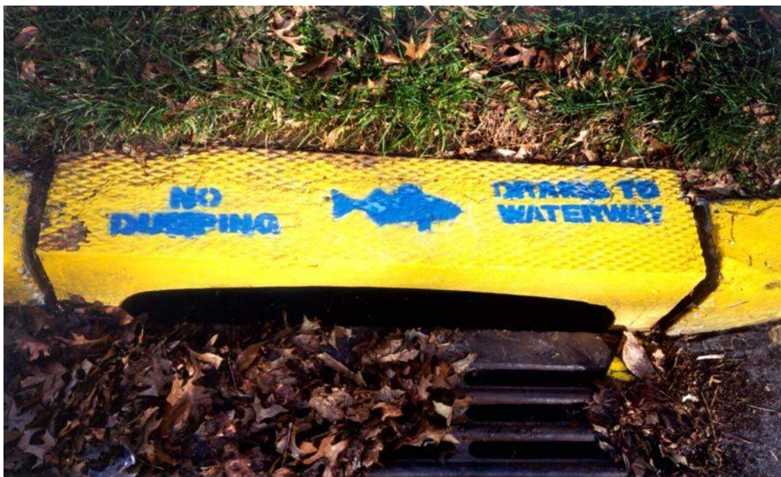
Storm Drain Catch Basin with stencil, Farnsworth Avenue
