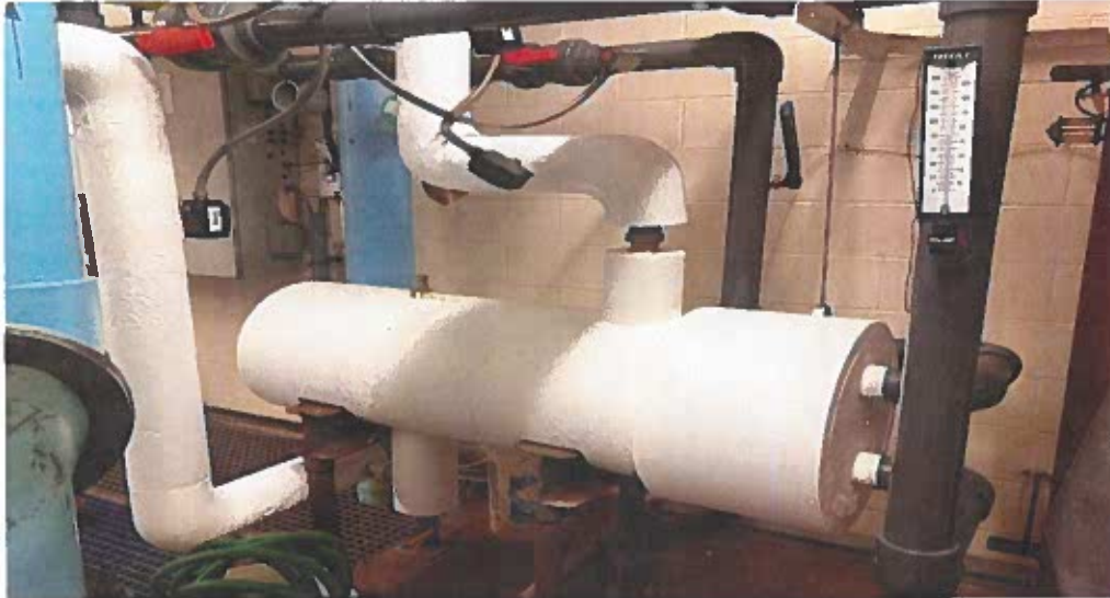
New pool heat exchanger located in the pool equipment room
