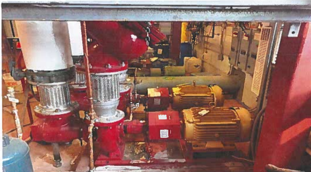
New boiler pumps and drives
