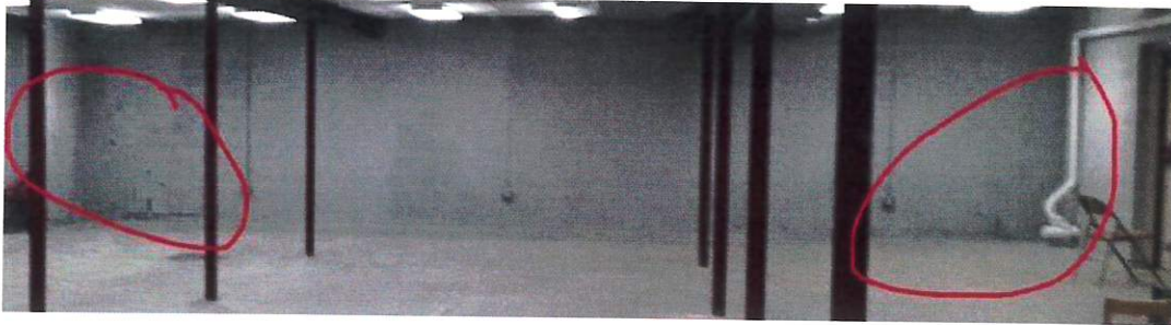
Fig. 2 Crack Locations - West Wall
