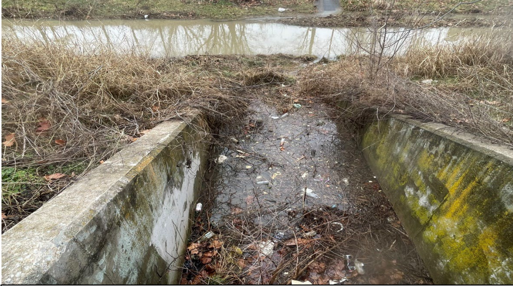
Figure 11. Storm drain outlet at the south end of Cleveland Street with large quantities of trash flowing directly into Spring Creek as well as impeding the natural flow of the drainage system itself.
