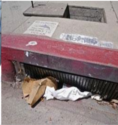
Figure 13. Curb Inlet Cover
