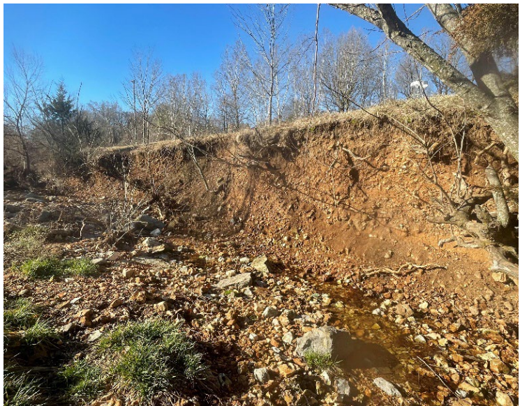
Figure 1. Severe/accelerated streambank erosion on spring-fed tributary just North of the Fleming Drive bridge, near J.B. Hunt Park
