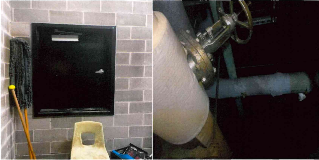
Entry Ways to North Crawlspace: The black door is on the main 1 st floor located on East end behind elevator area. The other access is in the boiler room North end. Asbestos Elbows in this area.
