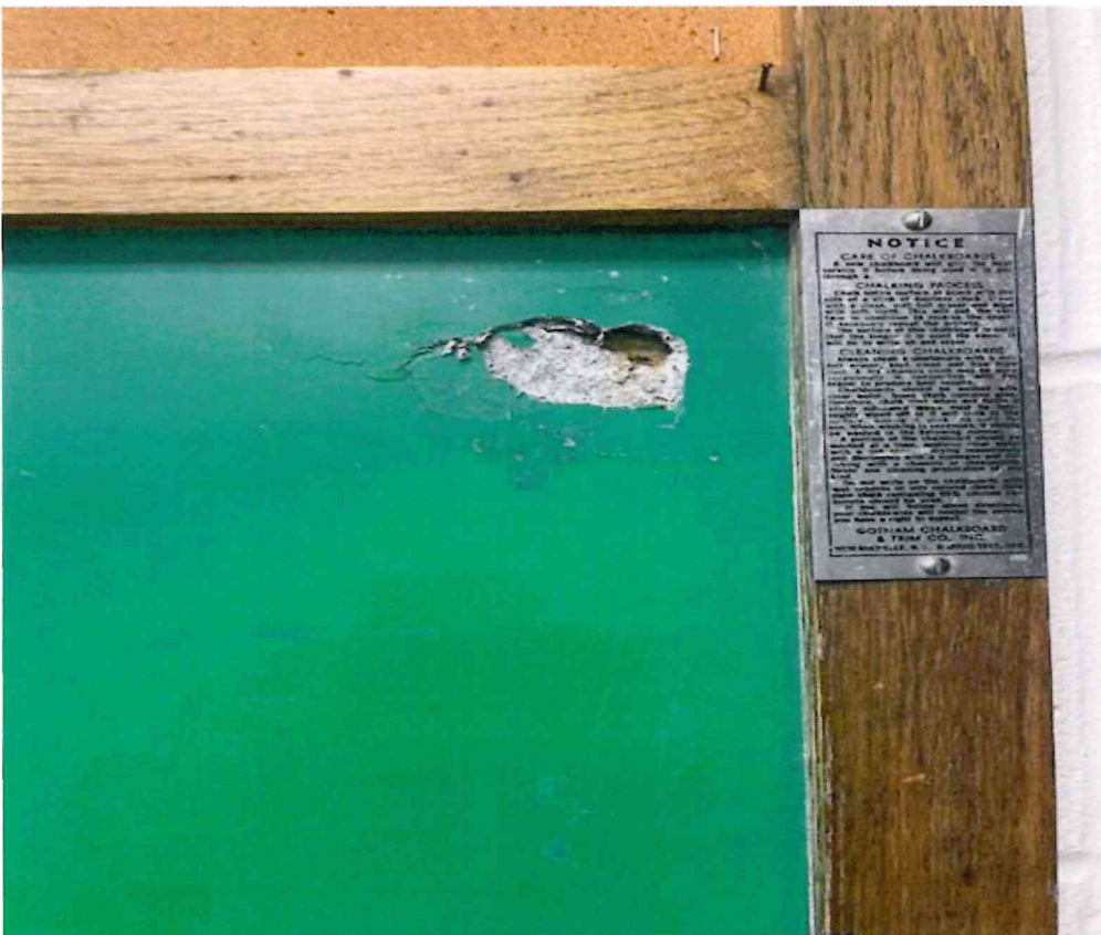
(11) Chalkboards with this label are containing 15% Chrysotile. Some of these chalkboards are covered with whiteboards or painted black
