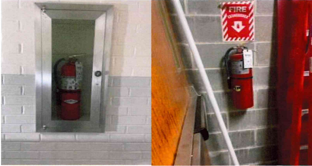
Items to remove or use in other locations: Several Fire Extinguishers
