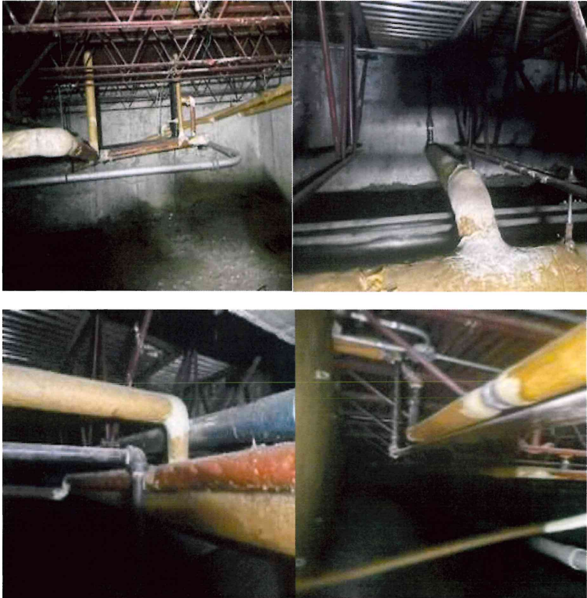
A few more pictures of North Crawlspace asbestos elbows/fittings.
