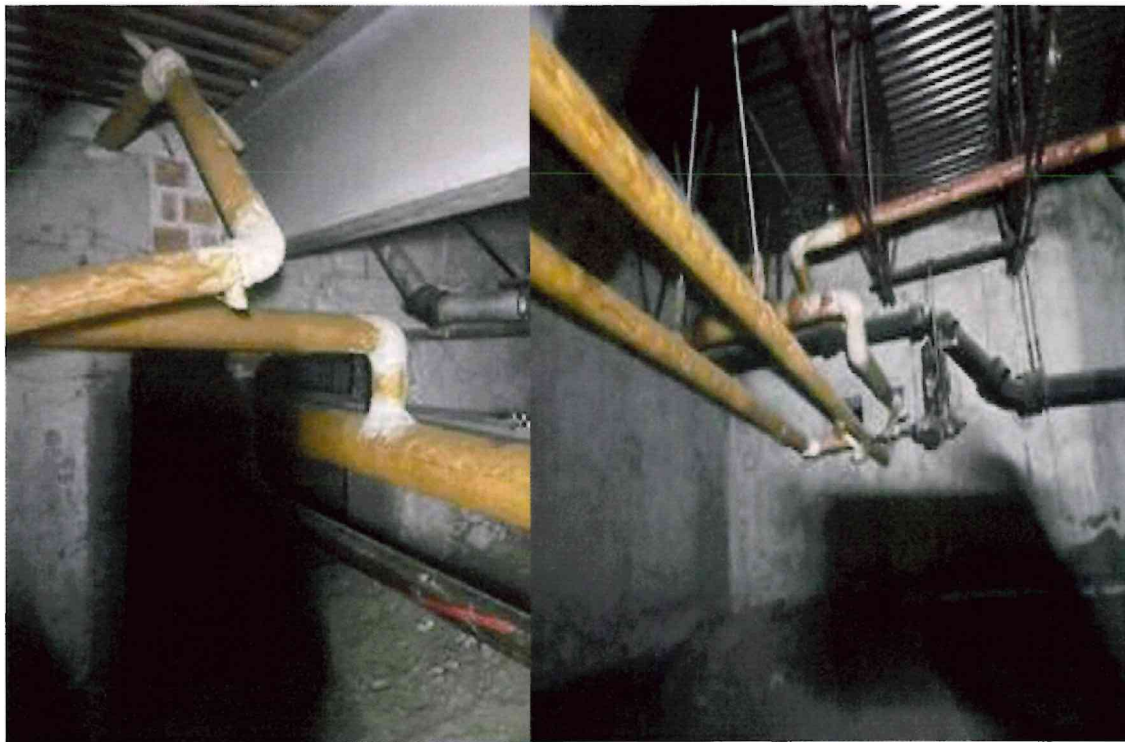
A few areas of the north crawlspace with asbestos elbows and fittings.
