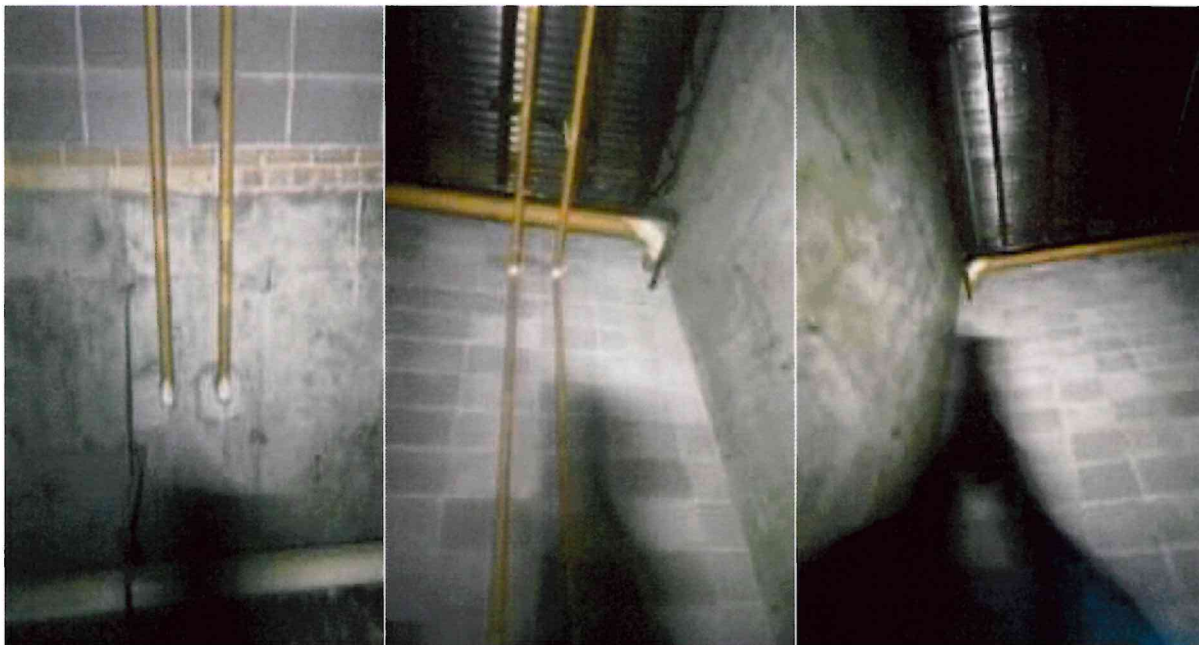
Elbows that are up high in the main North Crawlspace next to boiler room.
