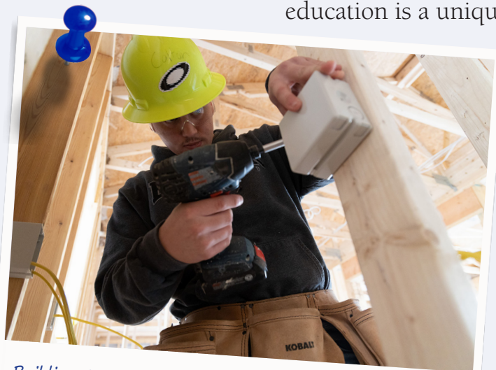
Building Construction student Colton Roark, from Poland Central School District, does drilling work inside the program's 42nd house during the 2022-23 school year.
