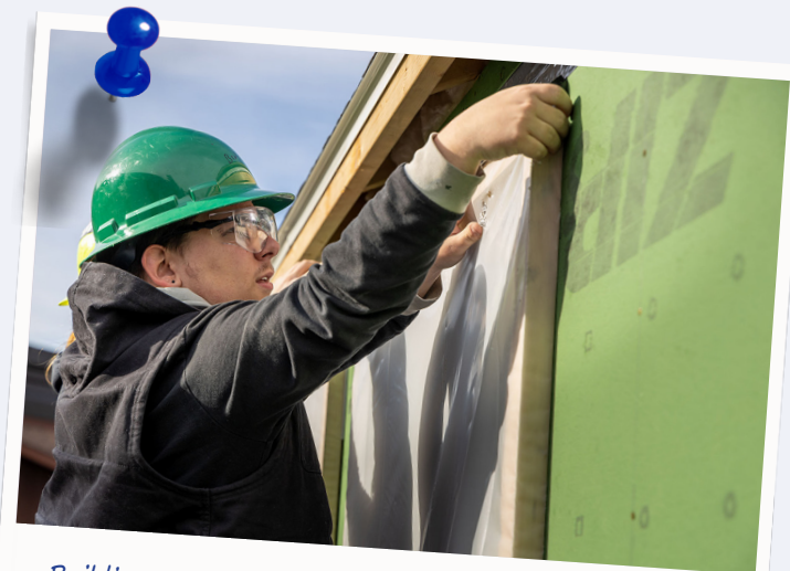
Building Construction student Brayden Hurteau, from Little Falls City School District, works on the outside of the program's 42nd house during the 2022-23 school year.
