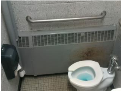
Rusted Radiant Heater
