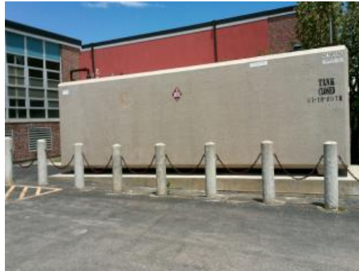
Fuel Oil Storage Tank
