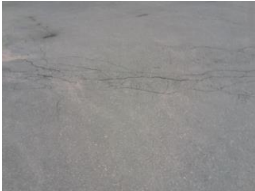
Worn Asphalt Parking Lot Pavement
