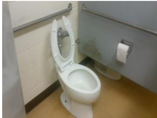
Rusted Toilet Partition
