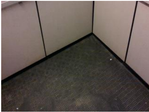
Elevator Floor Is Worn
