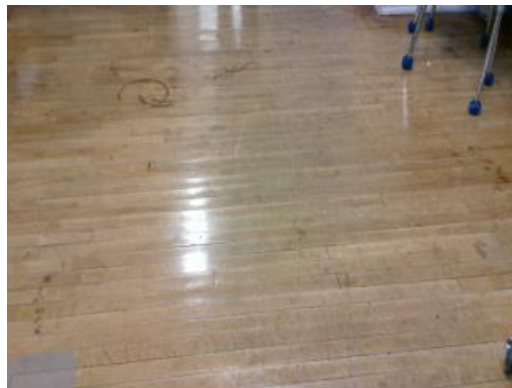
Worn And Scratched Wood Floor
