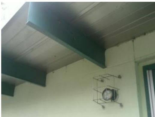
Paint Peeling At Canopies
