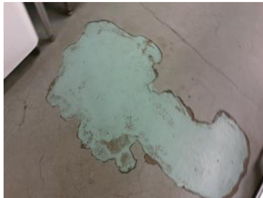
Damaged Epoxy Flooring In The Kitchen
