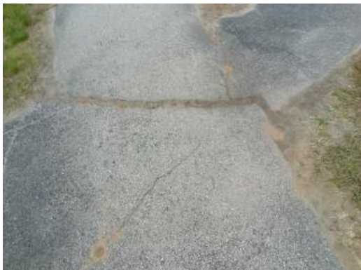
Weathered Asphalt Walkway
