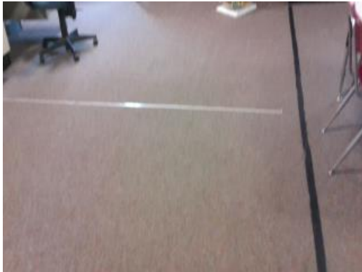
Damaged Carpet At Library
