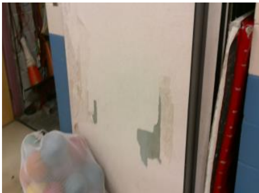
Damaged Movable Partition At Gymnasium
