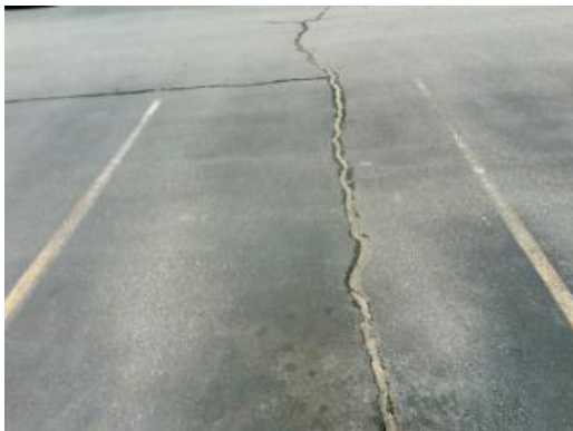
Weathered Asphalt Parking
