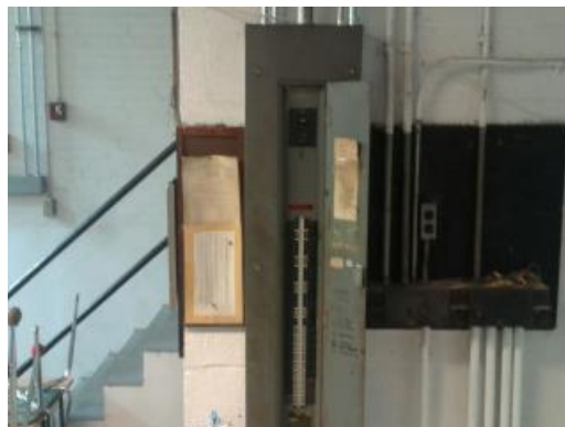
Federal Pacific Panelboard
