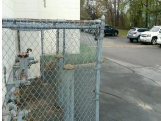
Damaged 8' Chain Link Fence
