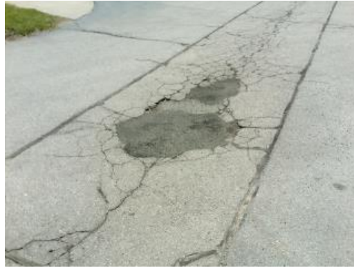
Alligatored Asphalt Pavement
