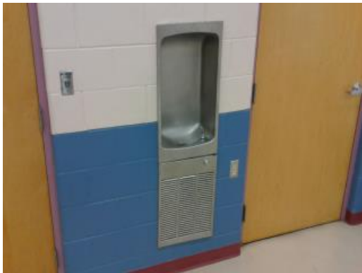
Refrigerated Drinking Fountain
