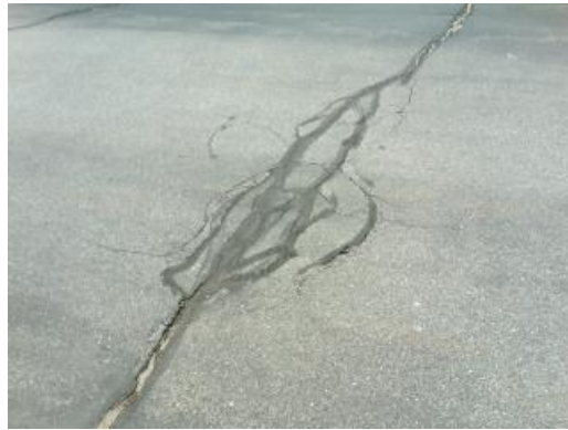
Cracked Asphalt Roadway
