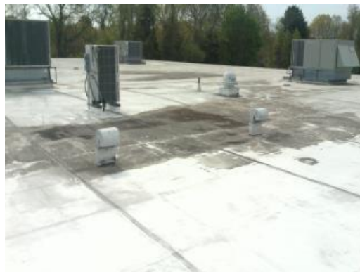
Ponding On Roof
