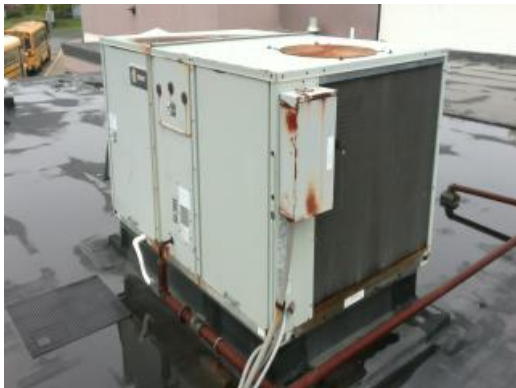
Rusted And Damaged Coils At Roof Top Unit
