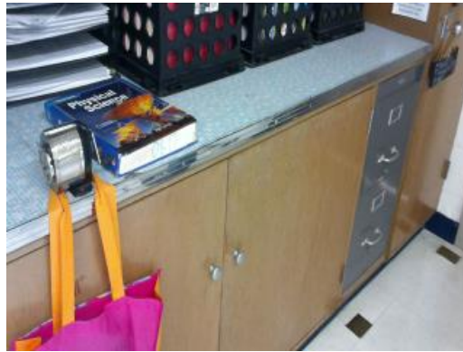
Peeling Laminate On Casework
