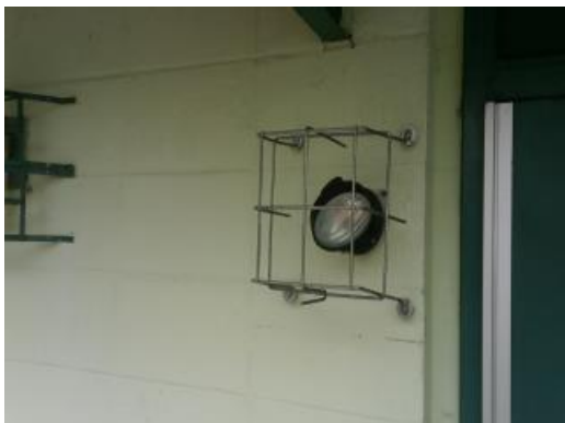
Aged Building Mounted Light
