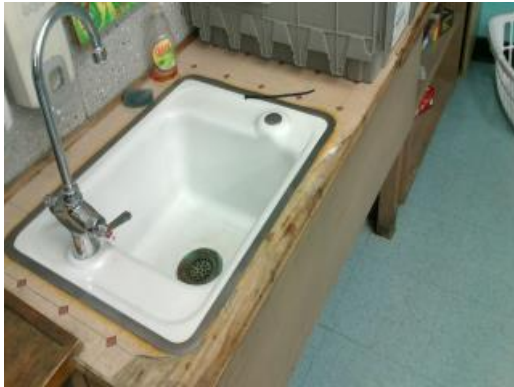
Damaged Classroom Cabinet
