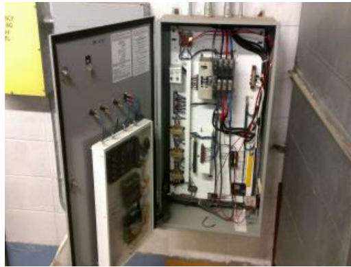
Automatic Transfer Switch
