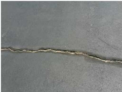
Cracked Asphalt Walkway
