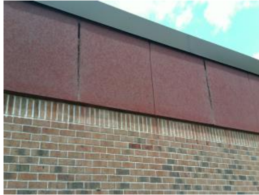
Weathered Caulking At EIFS
