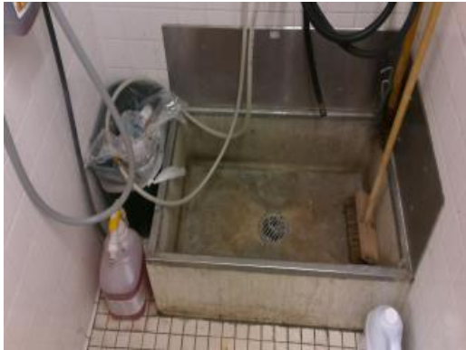
Rusted Mop/Service Sink
