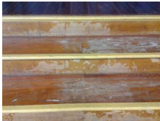
Damaged Wood Floor
