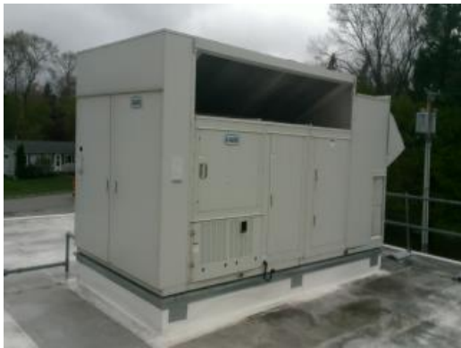
Large Energy Recovery Unit
