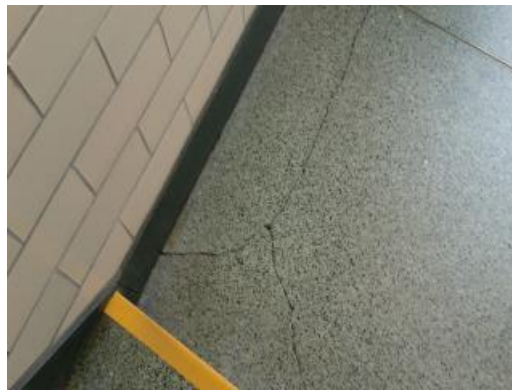
Cracked Flooring at Stairs
