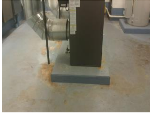
Worn Concrete Flooring
