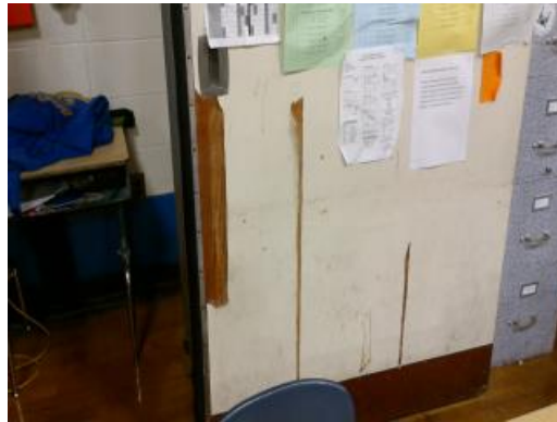
Damaged Moveable Gym Partition
