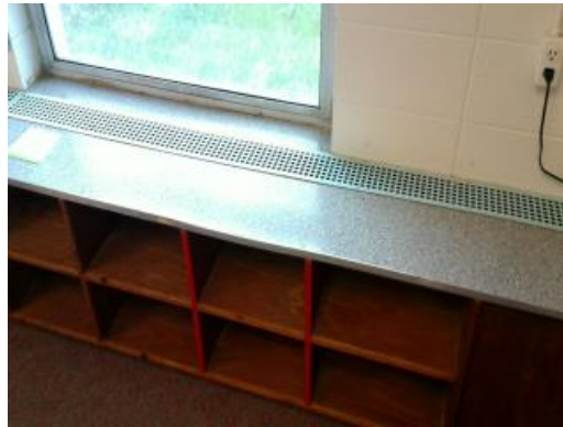
Clogged Coils And Rusted Casing At Fin Tube Heater
