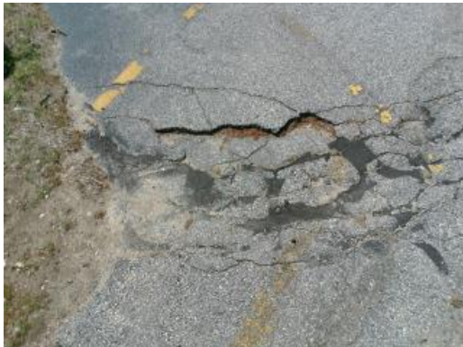
Deteriorated Asphalt Paving
