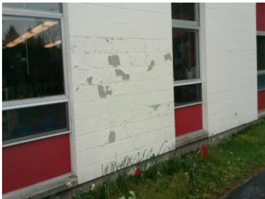
Peeling Paint At Exterior CMU Wall
