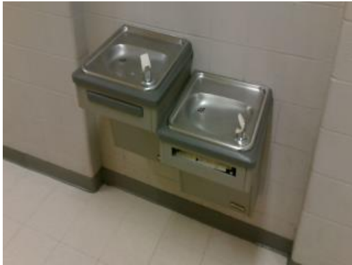
Non-Functional Refrigerated Water Fountains
