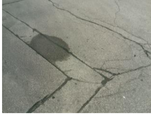
Typical Cracked Asphalt
