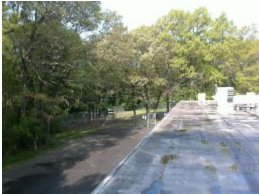
Weathered Roof With Ponding
