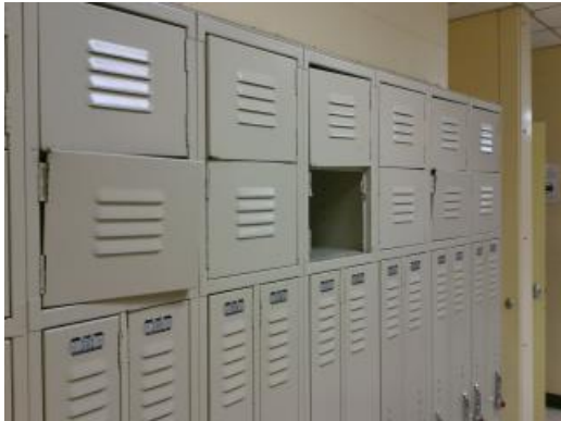
Lockers with Safety Concern at First Floor and Basement
