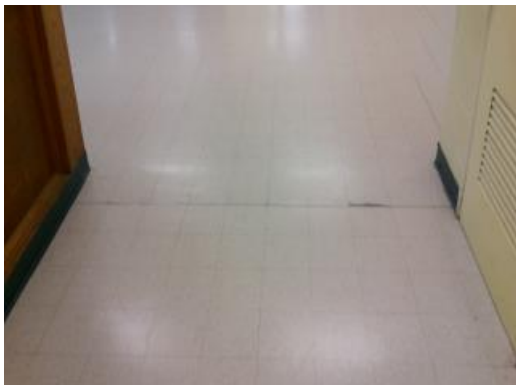
Cracked Flooring at Administrative Offices
