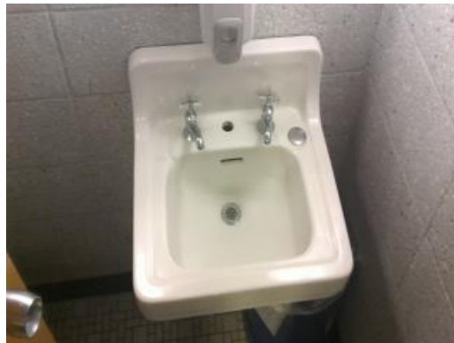
Typical Restroom Lavatory
