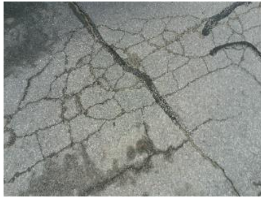
Cracked Asphalt At Roadway
