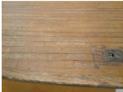
Worn Wood Floor
