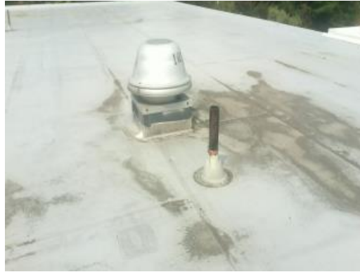
Evidence Of Ponding On Roof
