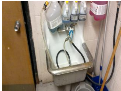
Stained And Rusted Mop/Service Sink
