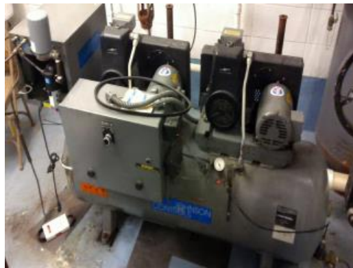
Inoperable Air Compressor
