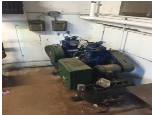
Leaking Air Compressor
