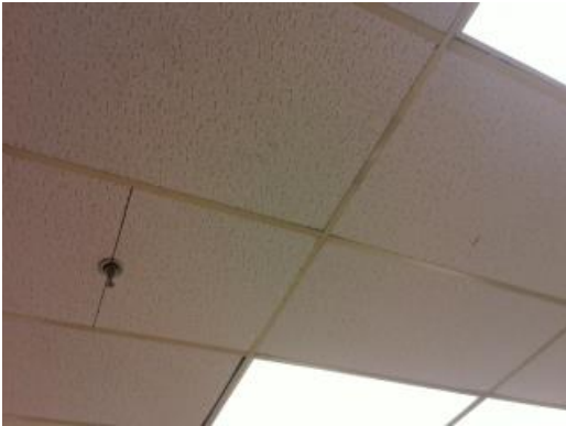
Stained Ceiling Grid
