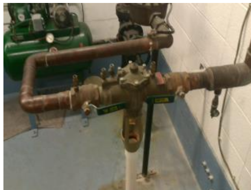
Corroded Backflow Preventer
