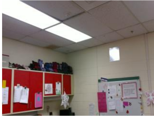
Stained And Sagging Ceiling Tiles
