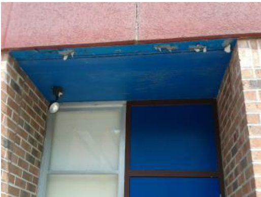
Peeling Soffit Paint
