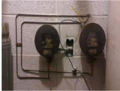
Aged Heating System Controls
