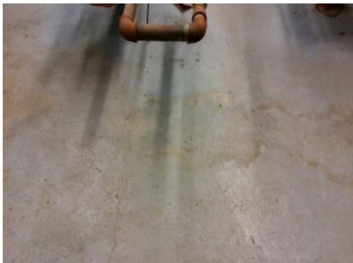
Concrete Finish Peeling At Boiler
