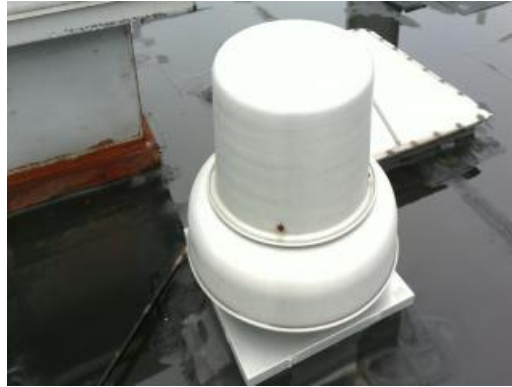
Rusted Exhaust Hood Casings
