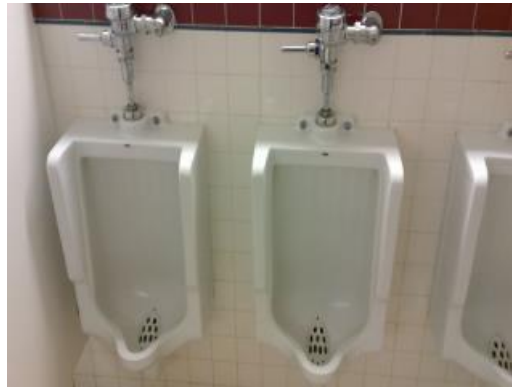
Stained And Corroded Flush Valves At Urinals
