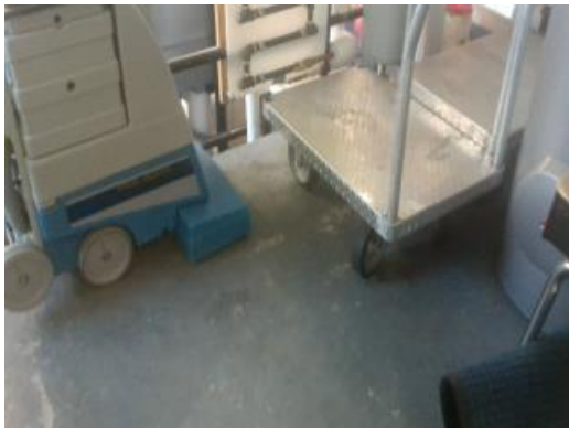
Worn Floor Paint
