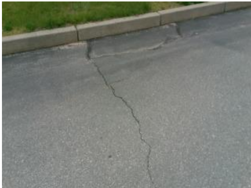
Worn Asphalt Roadway Pavement
