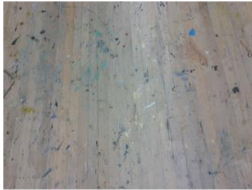
Damaged Wood Flooring At Stage
