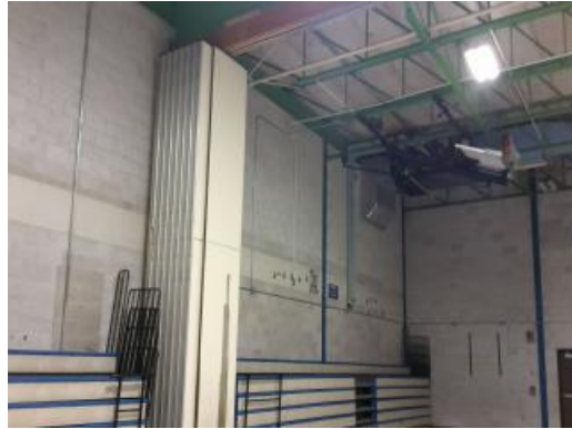
Damaged Gym Partition
