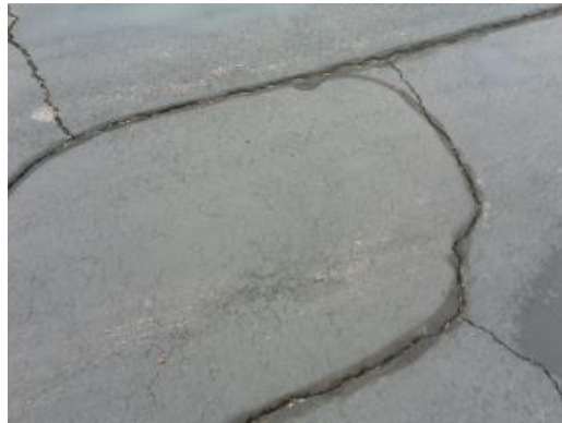
Roadway Asphalt Cracks
