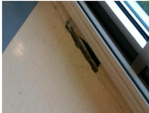
Cracked Flooring at Cafeteria
