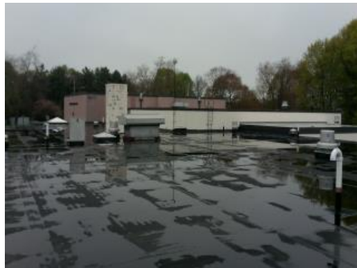
Damaged EPDM Roof
