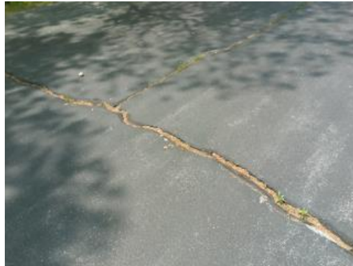
Cracked Asphalt Roadway
