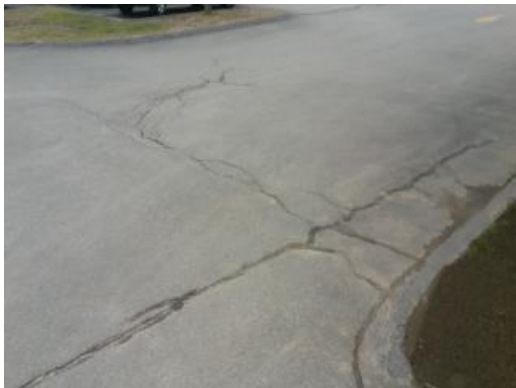
Damaged Asphalt Walks
