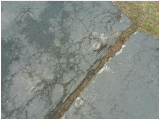
Parking Lot Cracks
