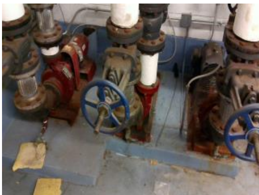
Rusted And Leaking Pump Seals
