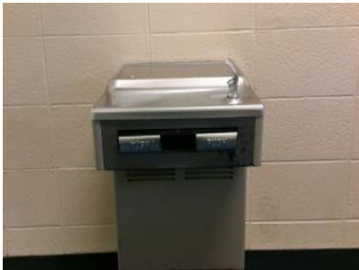
Damaged Drinking Fountain
