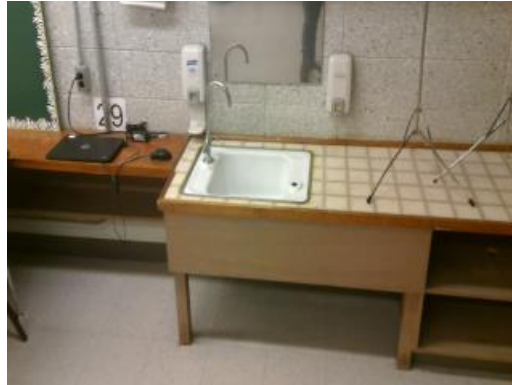
Aged Classroom Lavatory
