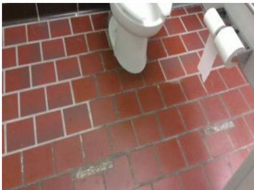
Cracked Ceramic Tile
