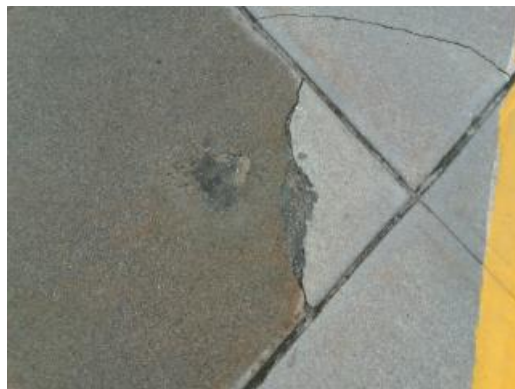
Cracking And Holes At Parking Lot
