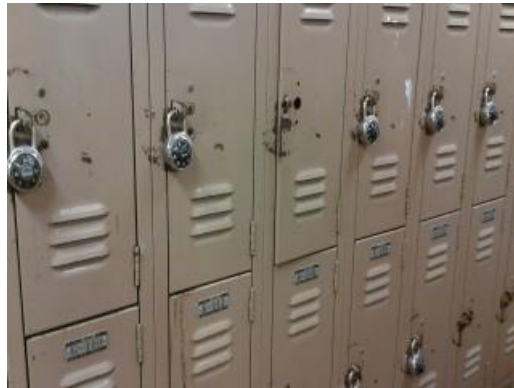
Corroded Lockers at Girls Locker Room
