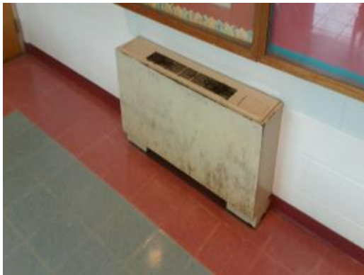
Clogged Coils And Rusted Casing At Unit Vent
