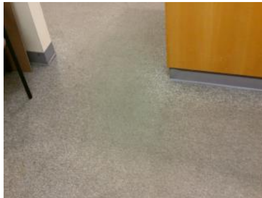
Worn Carpet At Main Office
