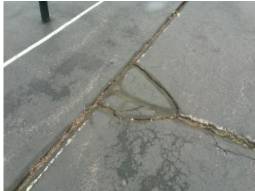
Cracking And Splitting At Play Area
