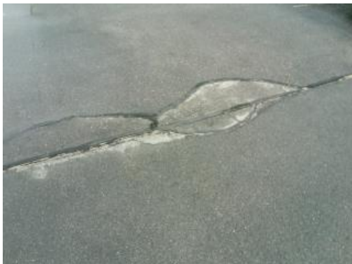
Cracked Asphalt At Parking Lot
