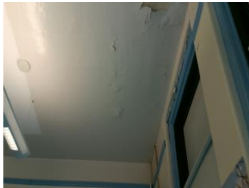
Peeling Ceiling Paint
