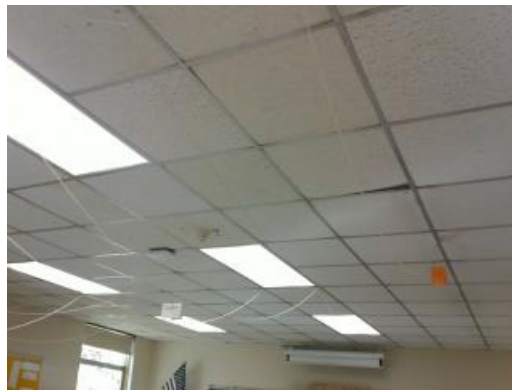
Aged and Damaged Ceiling Tile at Classroom
