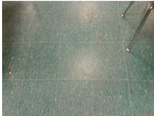
Faded And Worn VCT
