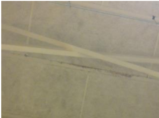
Damaged Tectum Ceiling in Gymnasium
