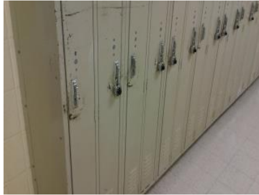
Corroded Lockers at Basement
