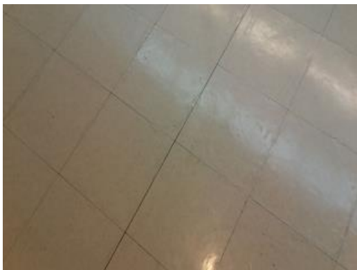
Damaged VCT By The Entrance Outside Gym 2
