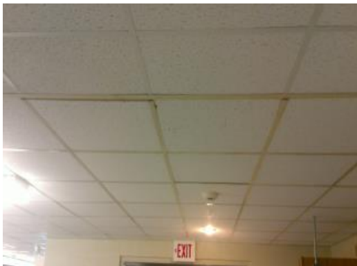
Stained And Broken Grid
