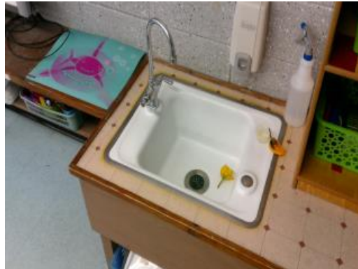
Damaged Classroom Lavatory
