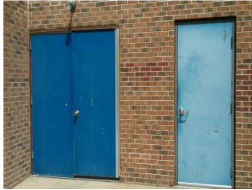
Aged Exterior Doors
