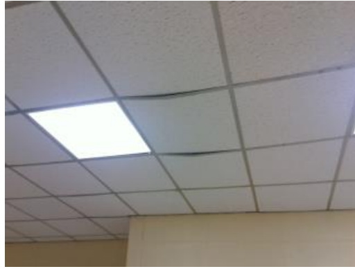
Damaged Ceiling Grid at Hallway
