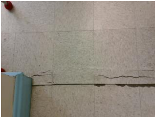
Cracked Flooring at Second Floor
