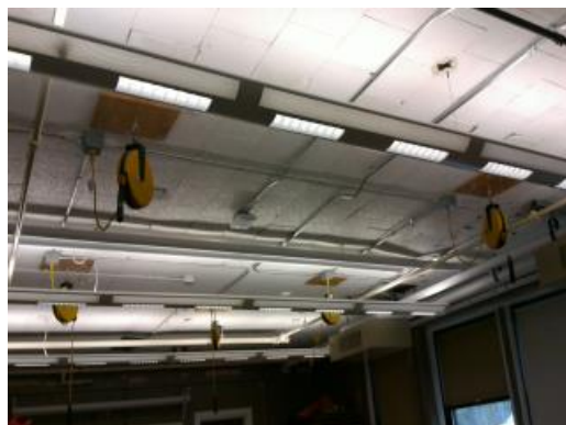
Falling Adhered Acoustic Ceiling Tiles
